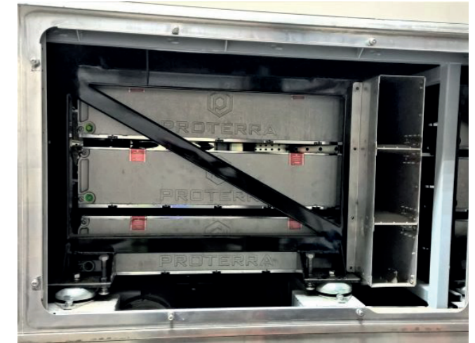
Battery Pack Ducts (access panels removed)
